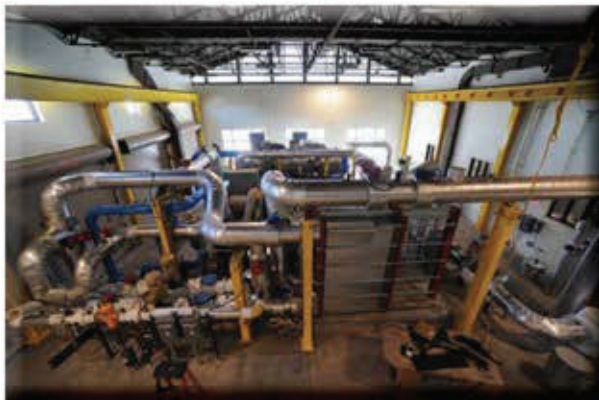
Fuel Gas Conditioning Unit
