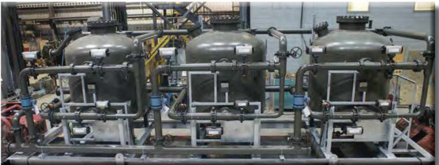
Filter Skid Assembly
